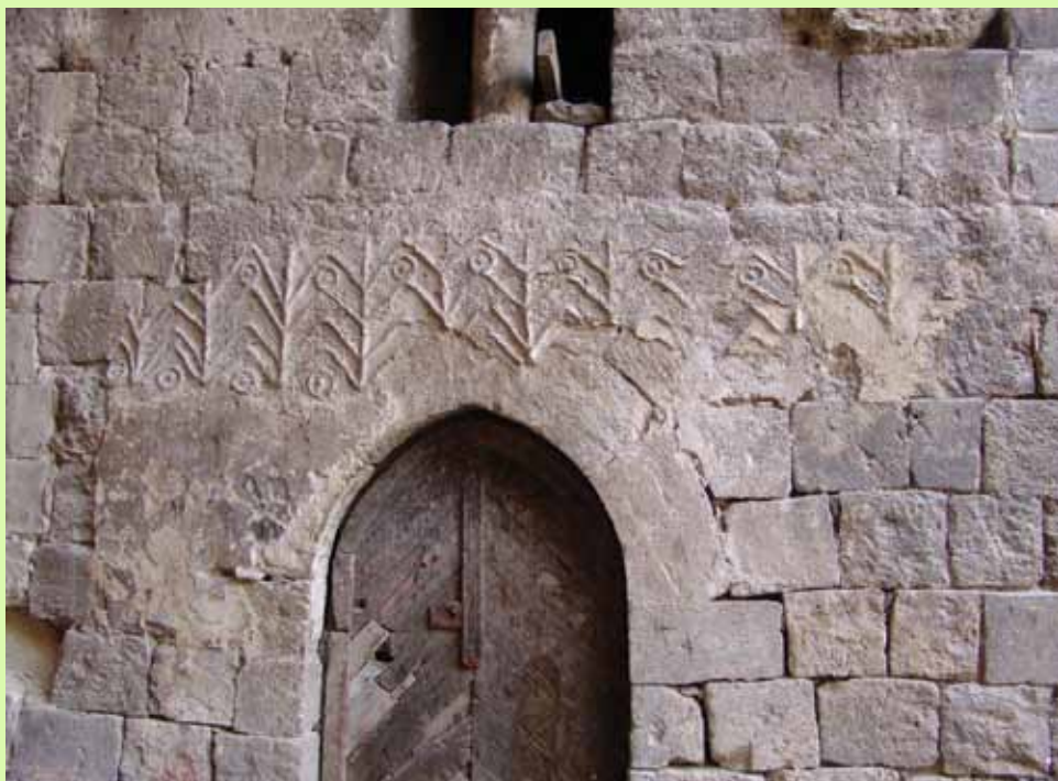
Detail from the traditional lime work in the Ottoman palace Dar al Kaid
