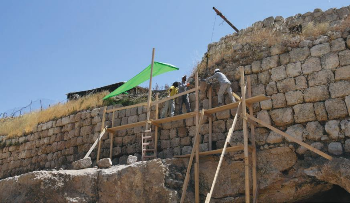
During the reconstruction and consolidation of the west wall of the Citadel.
