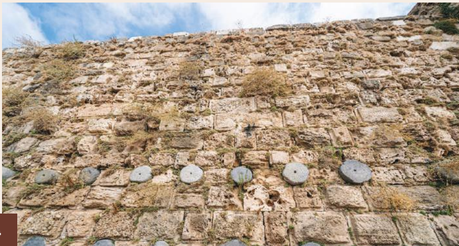
Detail of opus gallicum technique in the Byblos Crusader Castle in Lebanon
