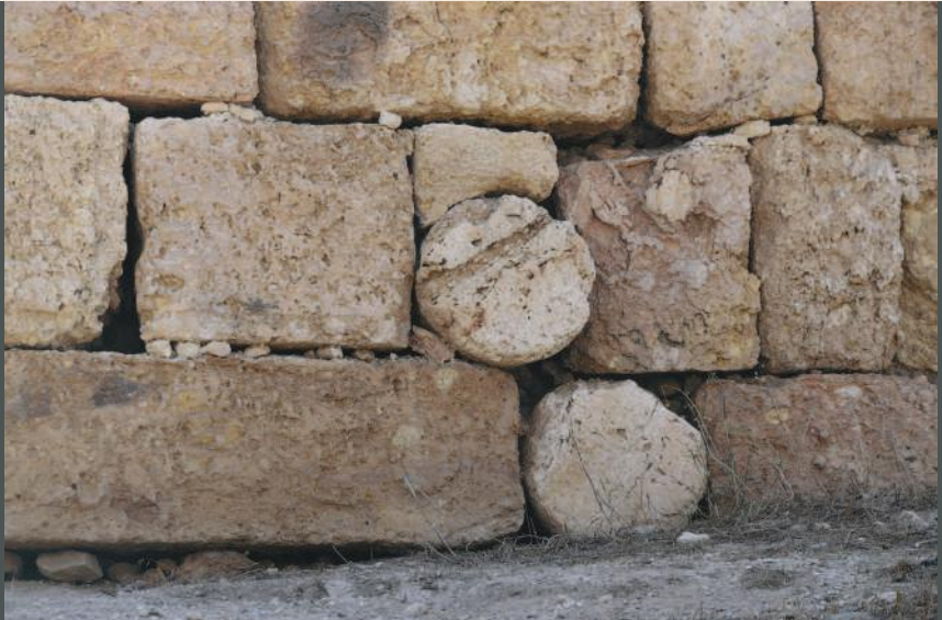
Detail of opus gallicum technique in the western wall of Al-Burj Citadel
